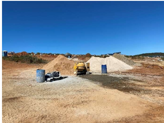
Cement washing spills at batching area within Phase 9.
