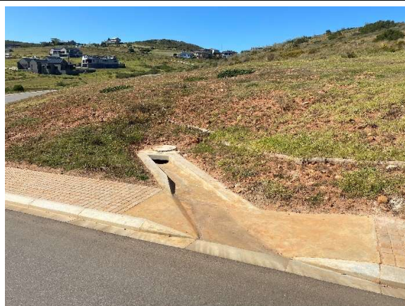
Stormwater infrastructure leading towards Phase 10.
