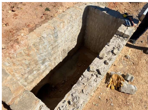
Stormwater infrastructure along the road.
