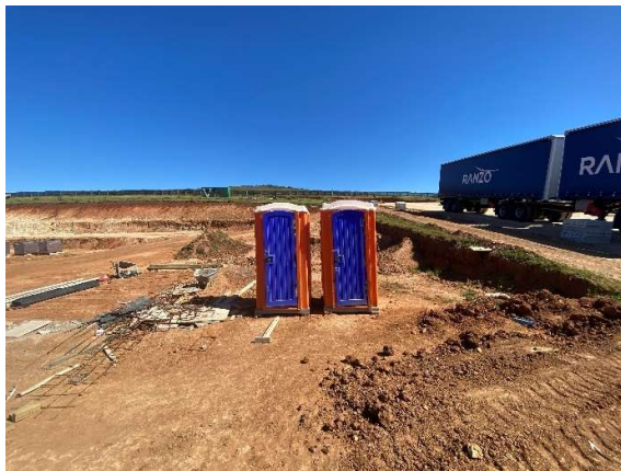
Chemical toilets available at the school construction site.
