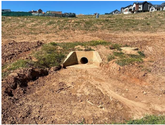
Stormwater outlet between Phase 4 and 9 directing stormwater towards the newly created detention swales.
