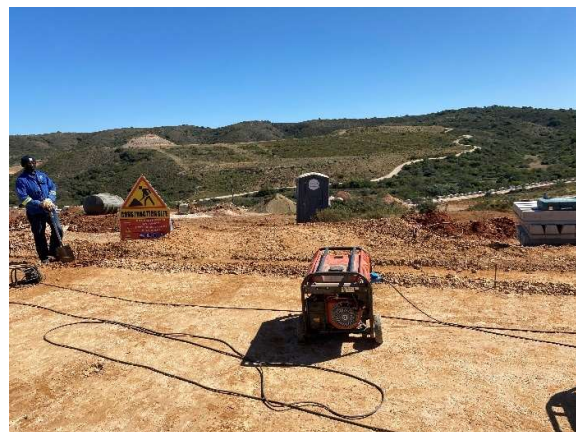
Generator present without a drip tray, but placed within the road footprint.
