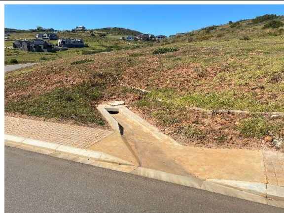
Stormwater infrastructure leading towards Phase 10.
