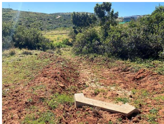
Stormwater outlet from Phase 9 into the natural stormwater valley.
