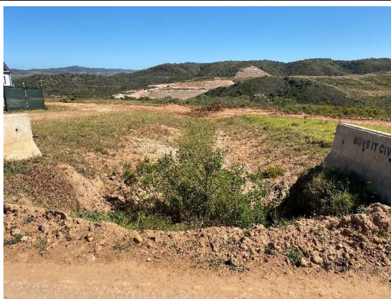
Stormwater outlet towards the retention pond north of phase 10.
