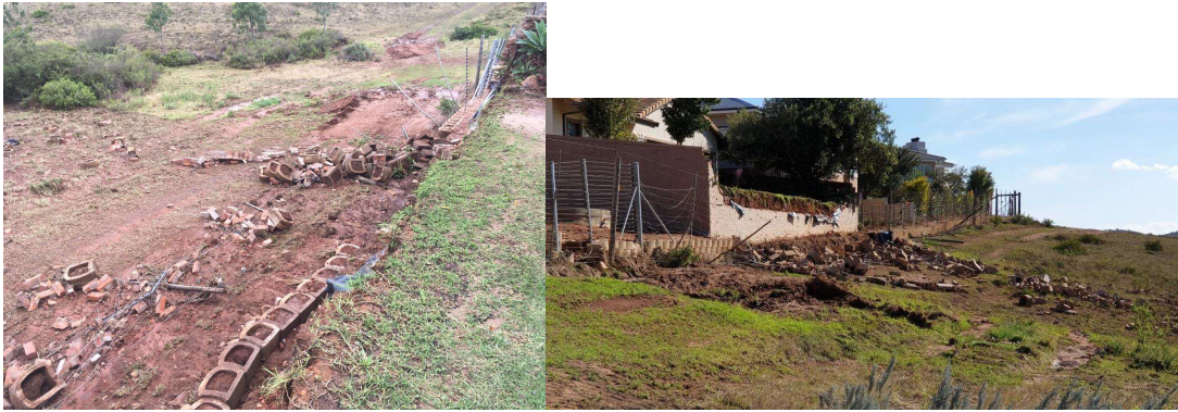
29 September 2019 storm damage from neighbouring Monte Christo estate – retaining wall collapsed onto the game fencing.
