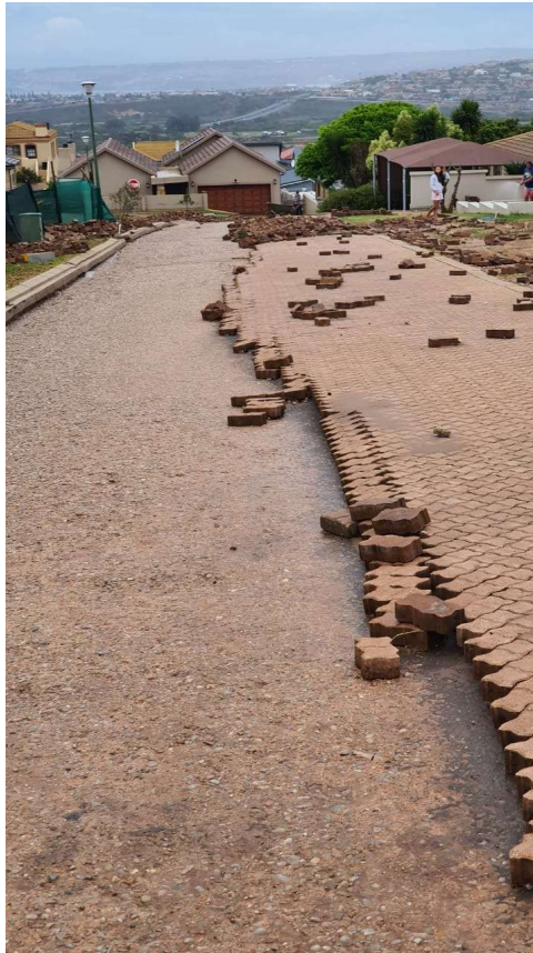
Storm damage to paved roads at neighbouring Monte Christo – resulted in the change in design of the roads from paving to asphalt surface.
