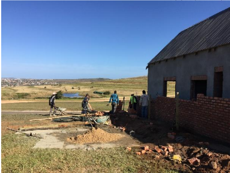
Construction rubble to be disposed of at an authorised waste disposal facility, and the area must be rehabilitated.
