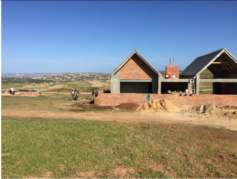
Construction material to be demarcated appropriately.
