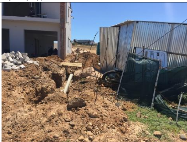
Open trenches must be demarcated to prevent accidental injury of animals (Erf 6644).
