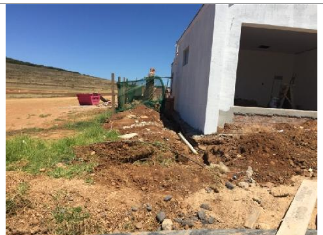
Open trenches must be demarcated to prevent accidental injury of animals (Erf 6557).
