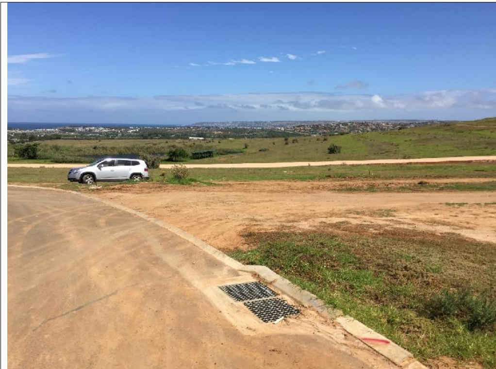
Temporary access road during the surfacing of the main access road must now be closed off and rehabilitated.
