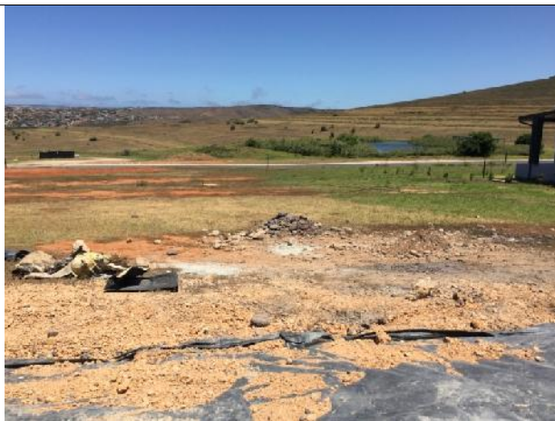
Sidewalk construction area must be cleared and rehabilitated.
