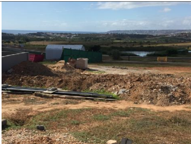
Construction material/soil must be demarcated (Erf 6619) (27.01.2021).
