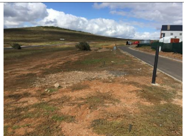
Concrete mixing area should be cleaned up and rehabilitated.
