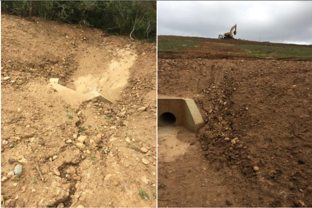
2021.11.05 – Stormwater outlet (phase 10) additional rehabilitation required - the estate management is busy with rehabilitation
