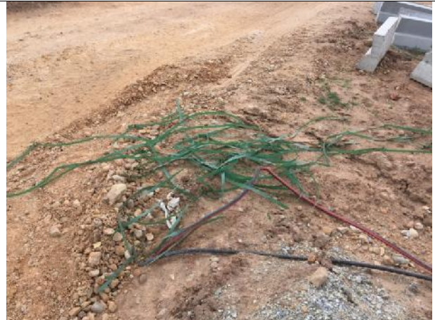
2021.11.05 – Litter must be picked up to prevent it from blowing around in the wind – was reported to the contractor and daily litter picking is done.
