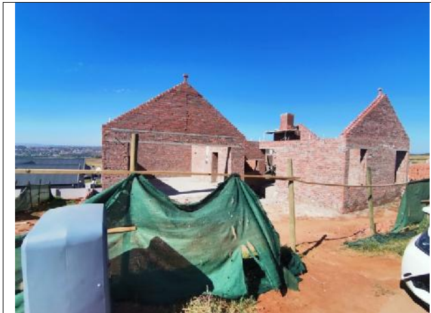
2022.02.02 – All properties must be fully demarcated with green shade netting.
