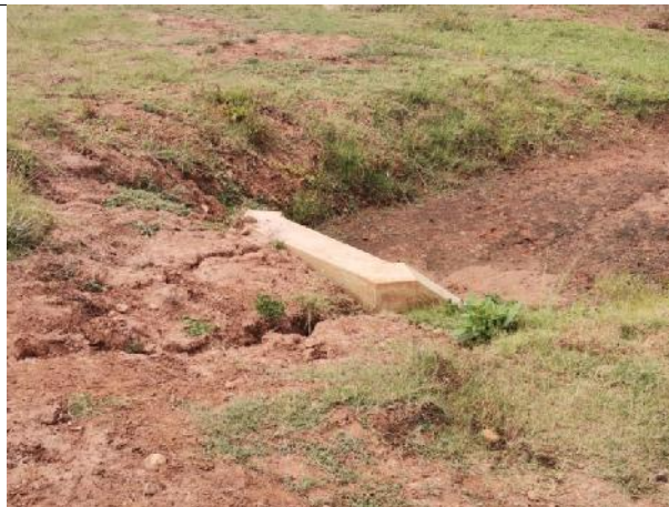
2022.01.27 – Stormwater outlet (phase 10) additional rehabilitation recommended (see Section 7) - the estate management is continuing with rehabilitation
