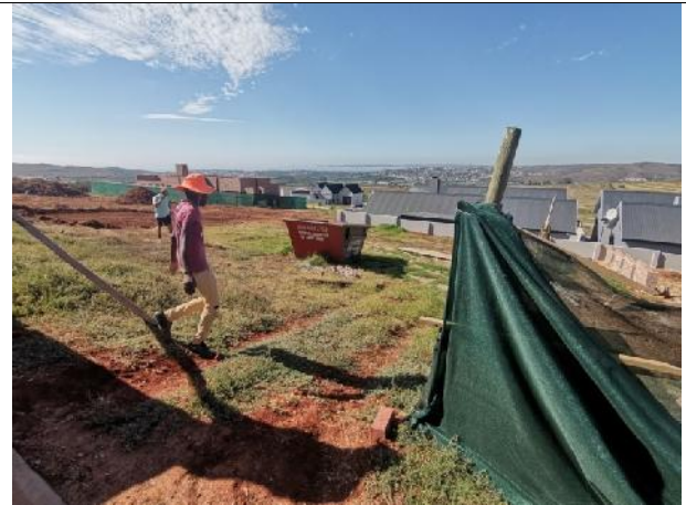
2022.02.02 – skip or litter bin must be covered to prevent litter from blowing away.
