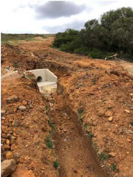
Silt fence required at the stormwater outlets
