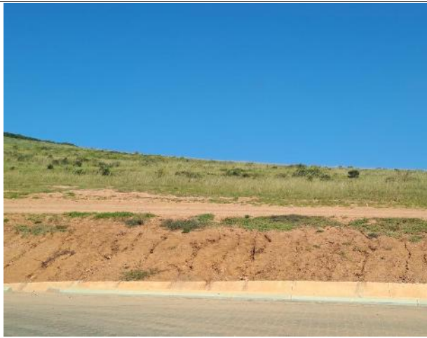
Erosion protection and rehabilitation required on steep slopes.
