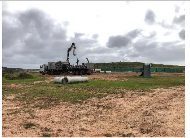
Material stockpile area (pipes etc.) is not fenced off. The contractor is required to fence off the material stockpile area as required in terms of the EMPr
