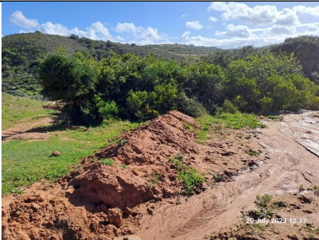
Small berm below outlet 6 – fix, replace topsoil, spread seed mix and vegetate. Note the silt buildup during construction phase in front of the berm – to be cleaned
