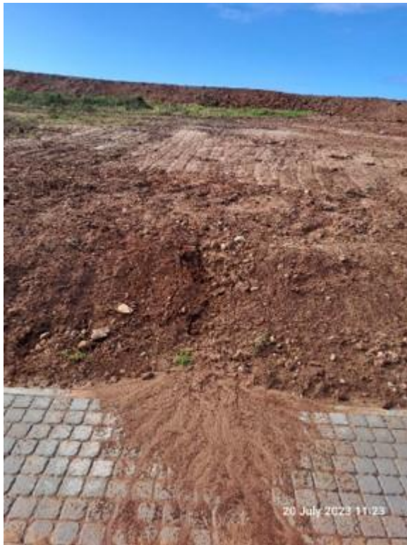
Road verge - steeper sections require erosion protection.
