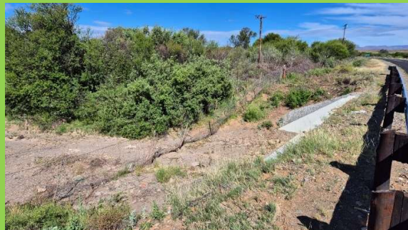
The ECO provided photographic proof on the 26th of November that the vegetation debris at the culvert (km38 on TR 16/9) has been removed.
