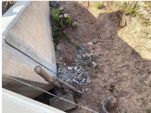
Cement and rubble observed in the riverbed at the Gabriel River bridge.
