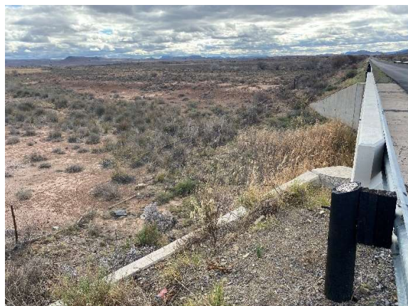
Downstream condition of the Brakvallei River bridge..
