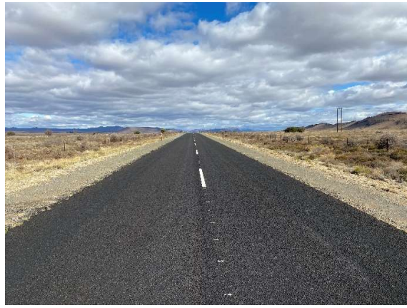
Condition of the road surface and the road reserve along the TR 16/9 as seen towards the southeast.
