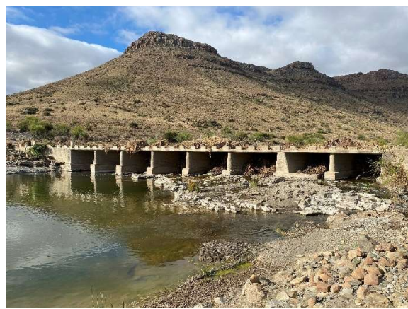
The old bridge which has been determined not safe for temporary traffic accommodation.
