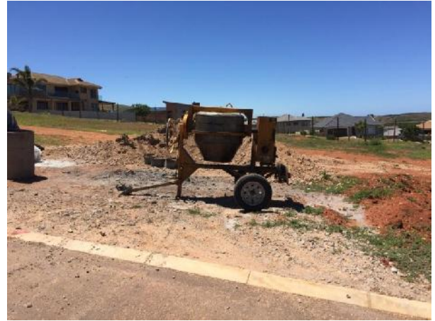
Concrete mixing should be done on a protective sheet with a small bunding wall to prevent contamination and possible run-off – the contractor was notified and the leftover concrete was removed.
