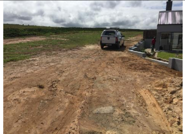
2021.03.17 - The temporary access roads adjacent erf 6557 MUST be closed off and rehabilitated.
