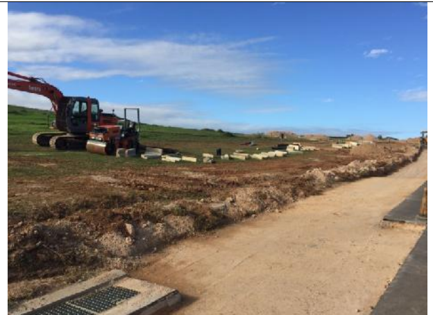
2021.04.28 – The areas currently used by the phase 3 contractor to store materials MUST be rehabilitated once they are done.
