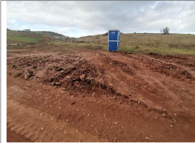
2021.06.23 – Phase 10 contractor providing a portable chemical toilet for the staff.
