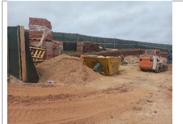
2022.09.29 – Skip available on site must be covered during inactive periods to prevent litter blowing in the wind.
