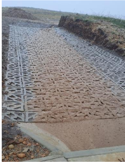
(2023.05.12) – Stormwater management (grass blocks) in phase 11 .
