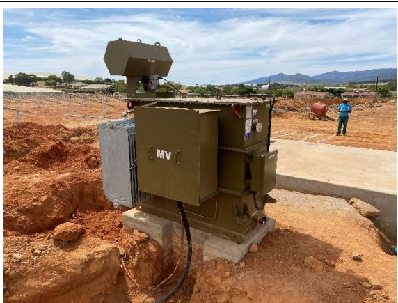
Completed electrical control stations.
