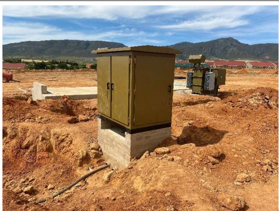
Completed electrical control stations.
