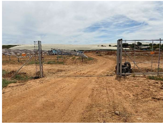
Entrance to the solar units.
