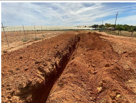
Groundwater cut-off trenches along the northern boundary conveying groundwater towards the west.
