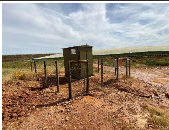
The ring main unit located immediately northwest of the site.
