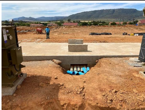
Electrical control station substructure.
