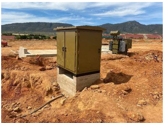
Completed electrical control stations.
