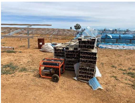
Structural material stored on-site with a generator. No drip tray in place.
