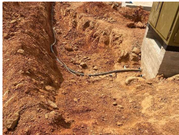
Installed electrical wiring leading from the solar panel units toward the electrical control station.
