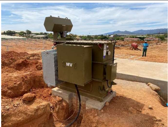
Completed electrical control stations.
