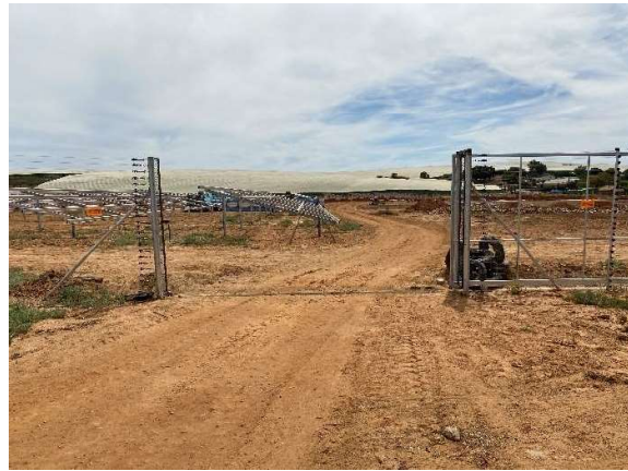
Entrance to the solar units.
