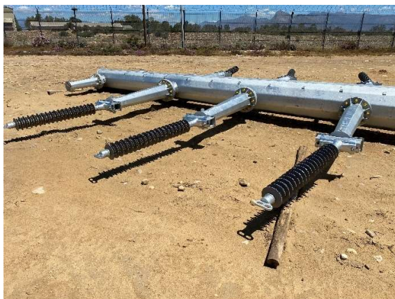
Pylon 4 per Figure 3 with porcelain insulator used to isolate the power wires at the edges.
