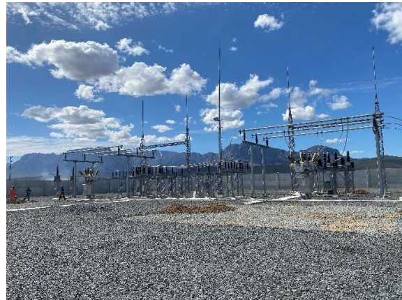
Within Transhex substation.
