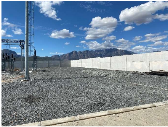
Within Transhex substation.
