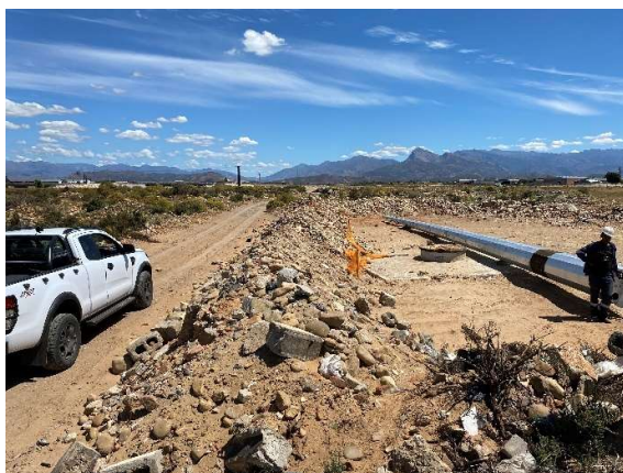
From pylon 8 as seen towards the south showing the derelict condition of this specific area.
