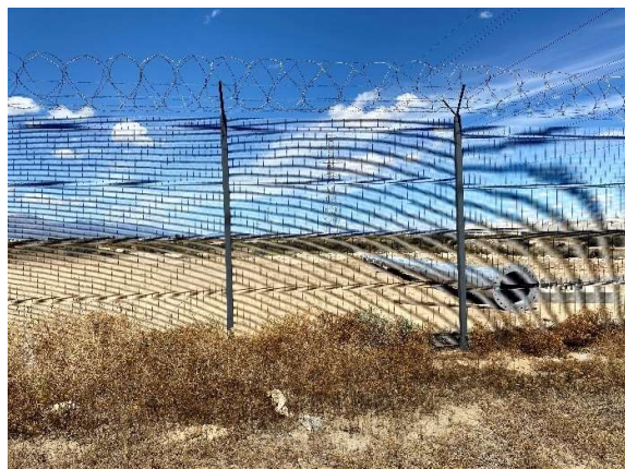
Worcester Industrial Substation boundary fence with pylon 3 in the back of picture within.
