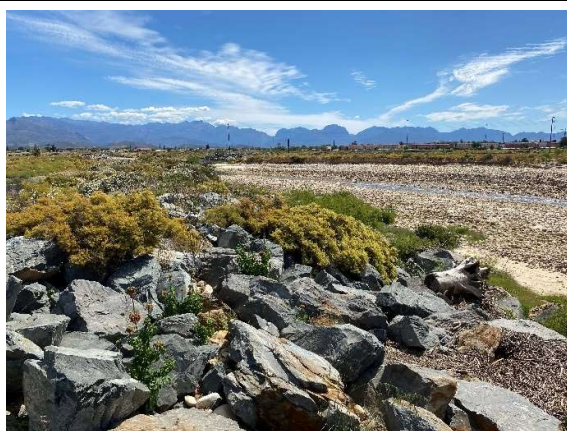
The condition of the Hex River and its banks immediately downstream of Robertson Road (R60).
