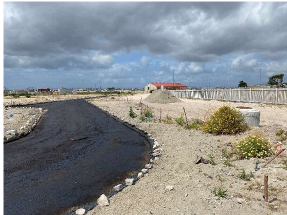
Condition of the recently surfaced internal road along the Sheffield road boundary with service manholes.
