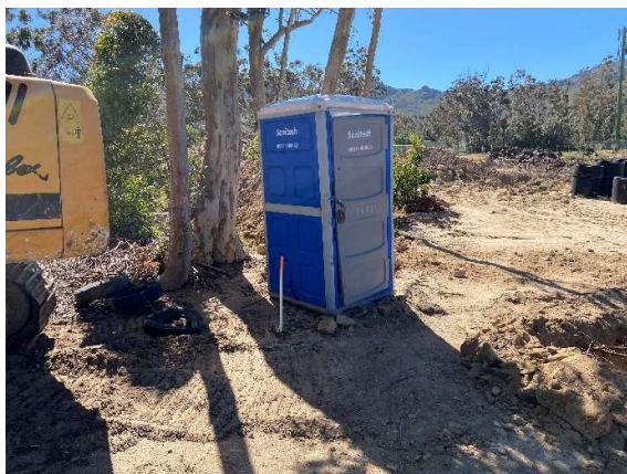
Additional chemical toilet present on-site adjacent to the contractors camp.
