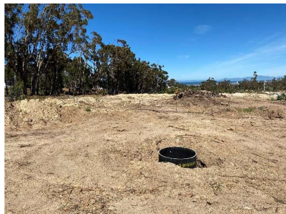
Service manhole in place at the southeastern corner of the site seen towards the west along the southern boundary.
