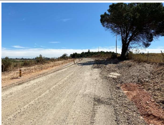
Condition of Protea Road as seen towards the west.
