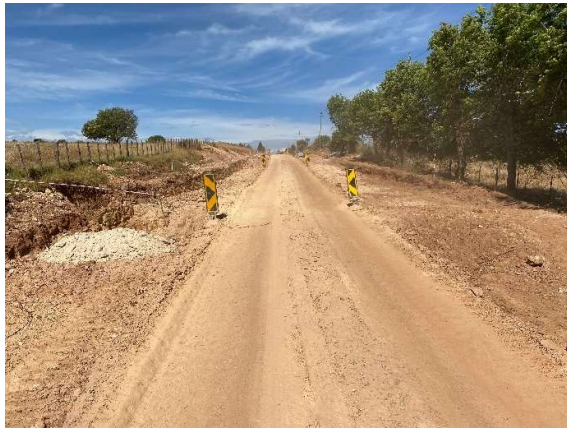
Condition of Protea Road as seen towards the east.
