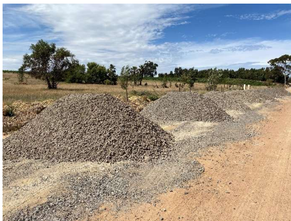
Current condition of Protea Road where aggregate is offloaded in place for the resurfacing.
