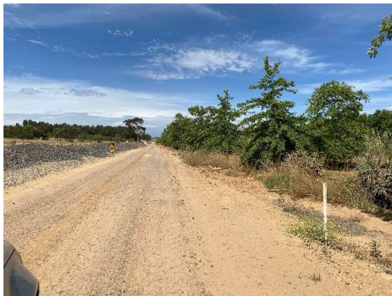
Current condition of Protea Road where aggregate is offloaded in place for the resurfacing.
