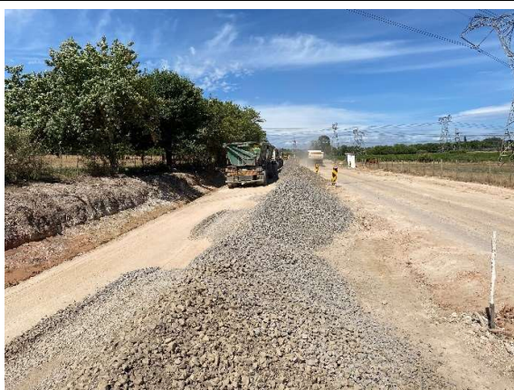
Condition of Protea Road where trucks are tipping aggregate in rows for halfwith construction.
