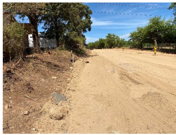
The condition of Protea Road along the Joostenberg Primary School.
