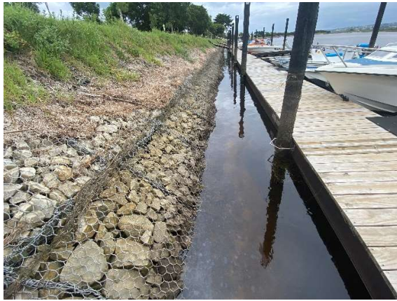
Reno-mattress toe at the bottom of the riverbank.
