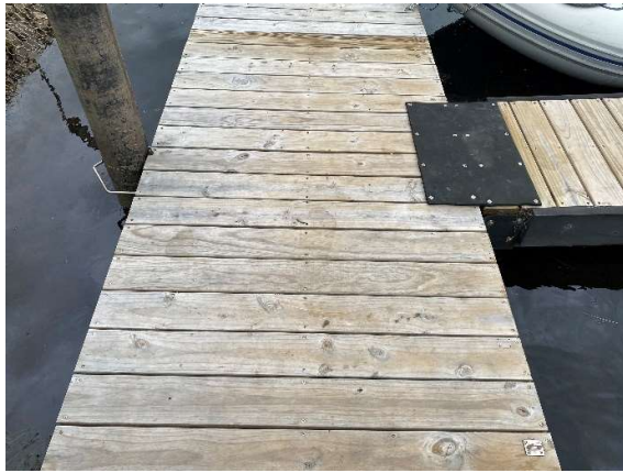
Attached floating jetty and mooring finger.
