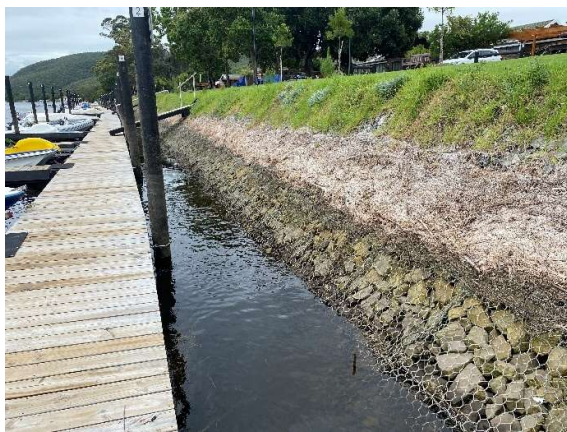
Condition of the jetty and the reno-matresses on low tide as seen towards the north.
