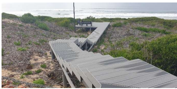
Condition of the broadwalk.
