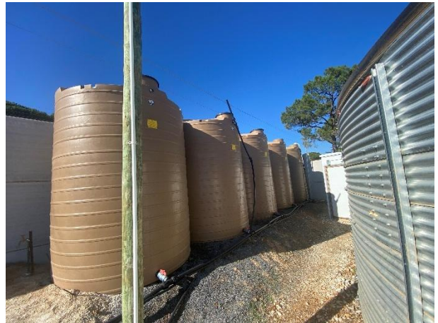
Jojo tanks and reservoir used for water storage (borehole).
