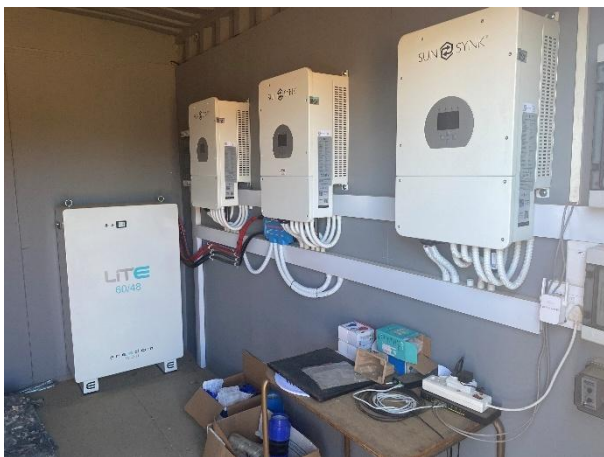
Locable container as the inverter room.
