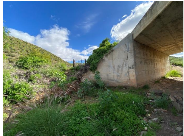
Repairs of vertical and horizontal cracks on the wingwalls.
