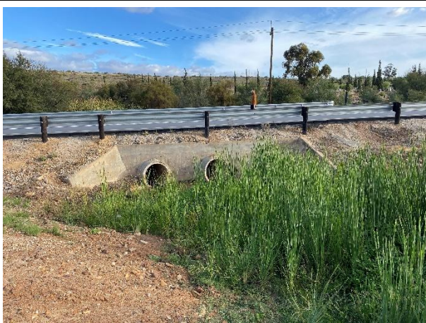
Overgrown vegetation due to the recent rainfall.
