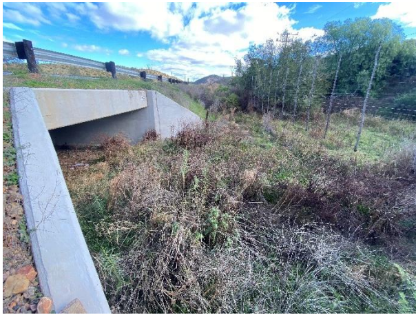
Overgrown vegetation due to the recent rainfall.
