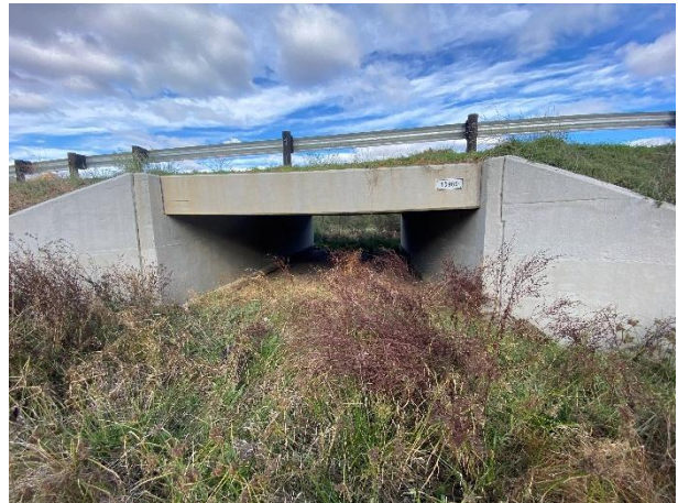
Overgrown vegetation due to the recent rainfall.
