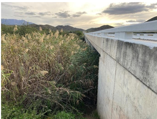
Overgrown vegetation due to the recent rainfall.
