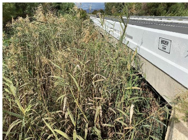
Overgrown vegetation due to the recent rainfall.
