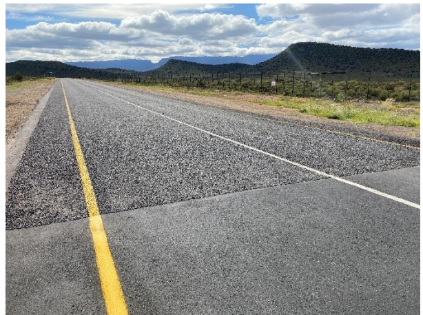
Condition of the road reserve and surface of TR 83/2.
