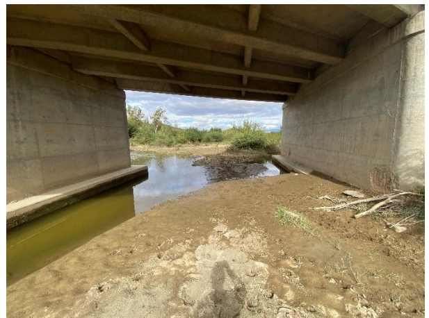
Removal of dense vegetation overgrowth and debris deposits.
