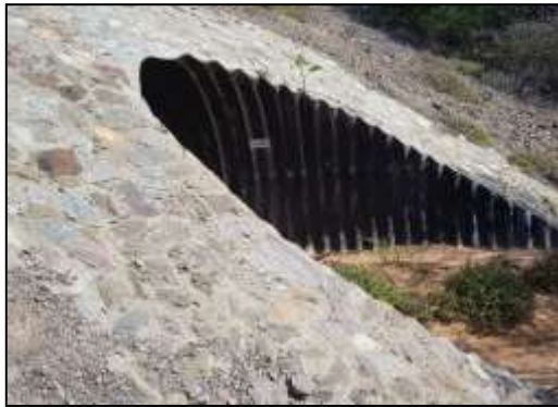
Figure 6: Large pipe culvert with headwalls and no apron slab.
