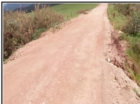
THE ROAD OVER THE CULVERT IS VERY NARROW AND ONLY ALLOWS FOR ONE WAY TRAFFIC. THE DROP OF THE CULVERT IS VERY HIGH AND POSE A HUGE SAFETY RISK FOR PEOPLE USING THIS ROAD.
