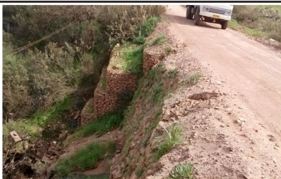
THE STRUCTURE OF THE CULVERT HAS BEEN SEVERELY ERODED AND DEGRADED AND URGENTLY NEEDS TO BE UPGRADED. EROSION IS AN ONGOING EVENT.
