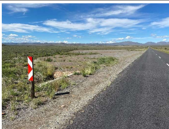
Condition of the road surface and road reserve along the TR 16/9 as seen towards the southeast.
