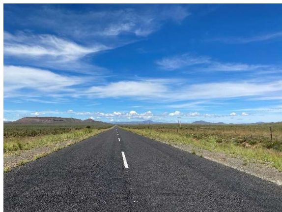
Condition of the road surface on TR 16/9.
