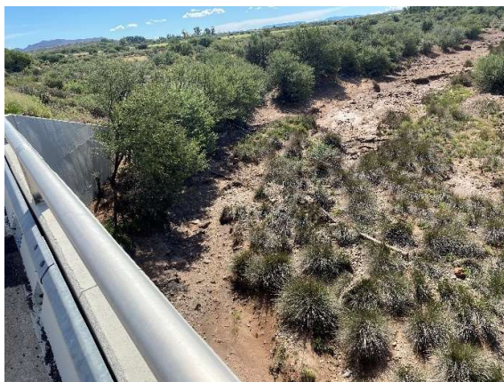
Upstream condition of the Brakvallei River bridge.
