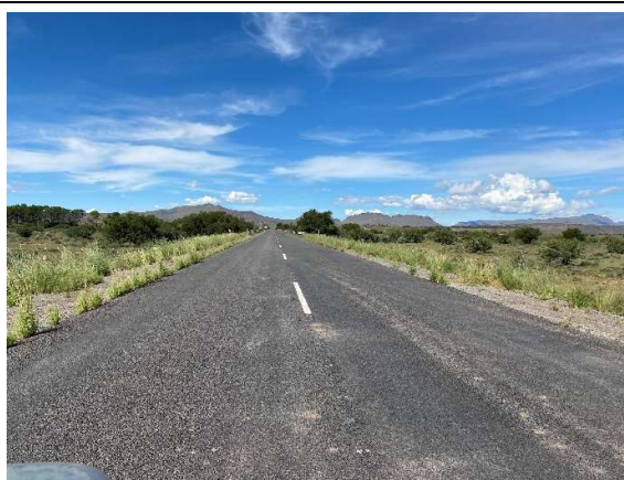
Condition of the road surface and the road reserve along the TR 16/9 as seen towards the southeast.
