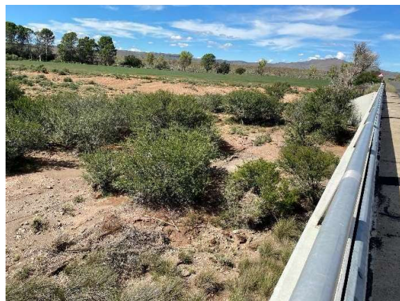
Downstream condition of the Brakvallei River bridge..
