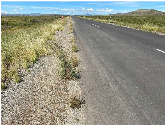
Condition of the road reserve on TR 16/9.
