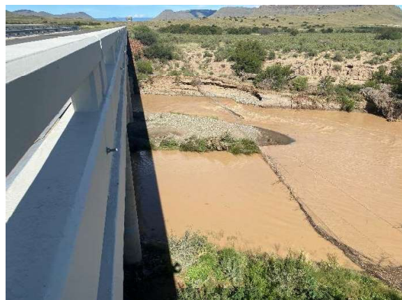
Condition downstream of the Buffalo Bridge.
