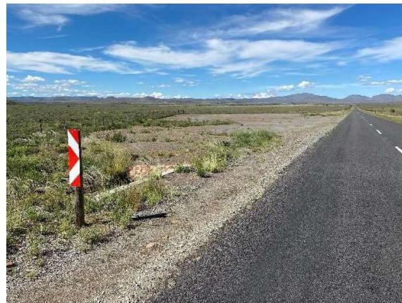
Condition of the road surface and road reserve along the TR 16/9 as seen towards the southeast.
