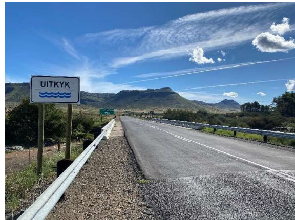
Condition of the Uitkyk Bridge.
