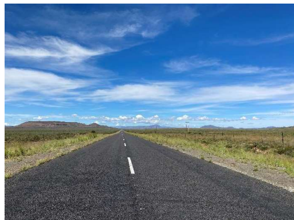
Condition of the road surface on TR 16/9.
