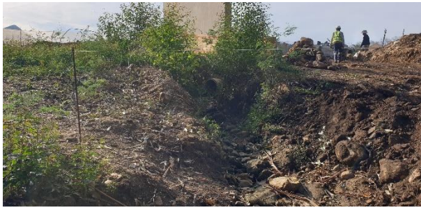
Stormwater outlet towards the riparian area.
