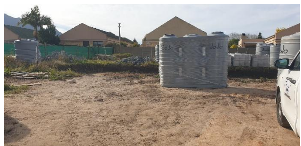
Jojo tanks are to be installed at each unit.
