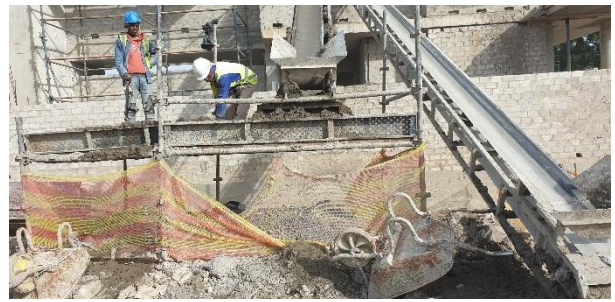
Cement conveyor belt, demarcation around the area.
