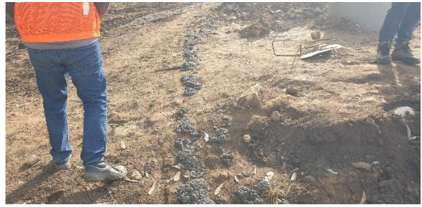
Cement spills adjacent to the rehabilitation area and stormwater outlet.
