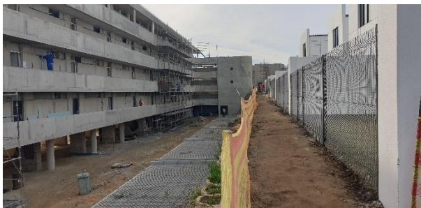
Demarcation netting is installed to prevent contractor falls at edges.
