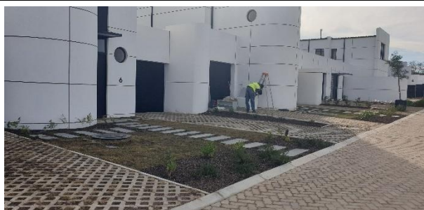
Permeable paving "grass block", SUDS intervention.
