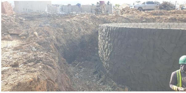
Cement batching in progress without the necessary mortarboards or drip trays.
