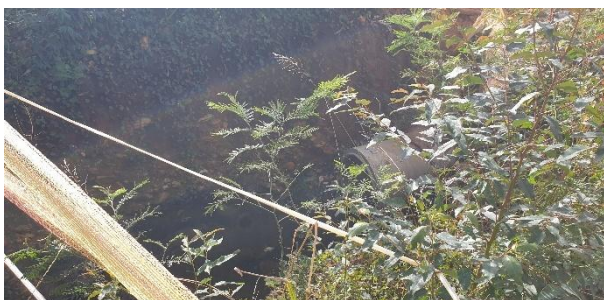
Stormwater outlet towards the riparian area.
