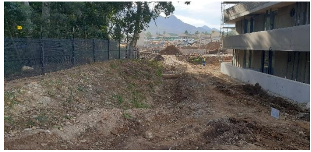
Temporary stormwater channels for surface flow.
