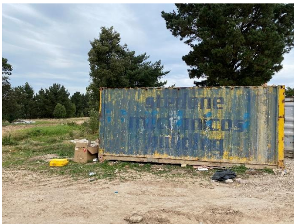
Lockable storage container in place near the next phase of the development, where services are being installed.
