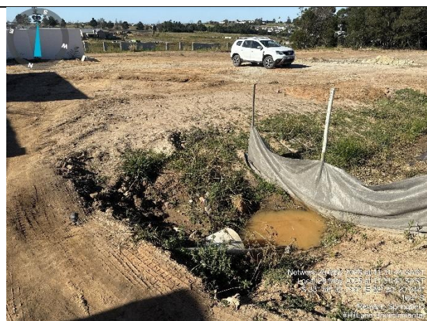
Silt fences are in place and must be maintained.
