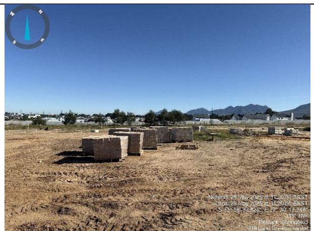
Construction material in the development area. Note the disturbed areas will need to be rehabilitated before final completion.
