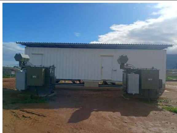
Completed electrical control stations.
