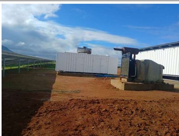
Completed electrical control stations.
