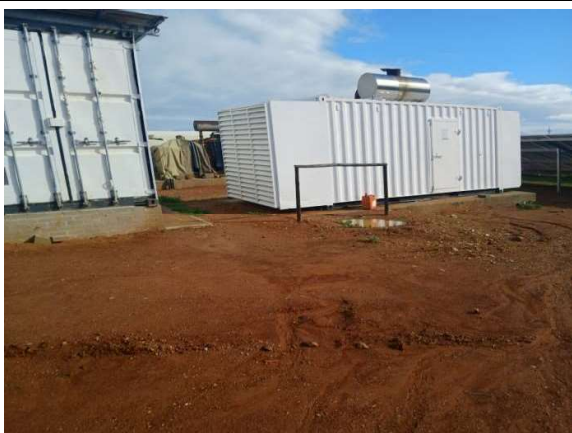
Completed electrical control stations.
