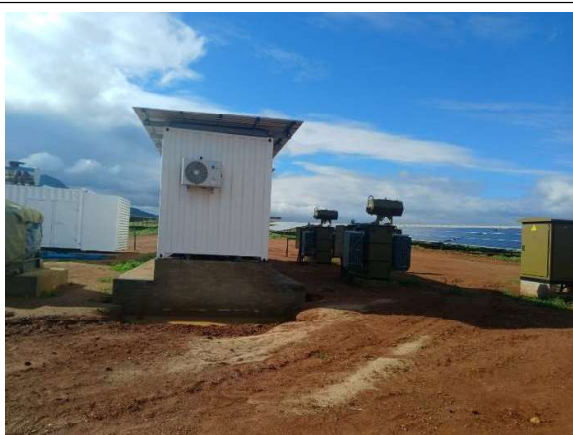
Completed electrical control stations.
