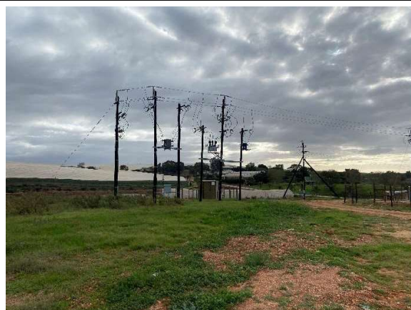
The ring main unit located immediately northwest of the site.
