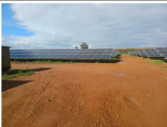
Solar panels as seen from the centre of the site towards the south.
