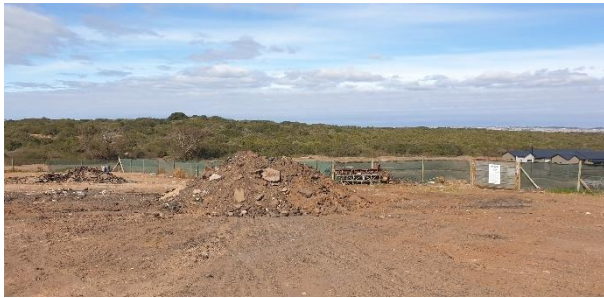
Condition of the construction camp adjacent to Erf 7380.
