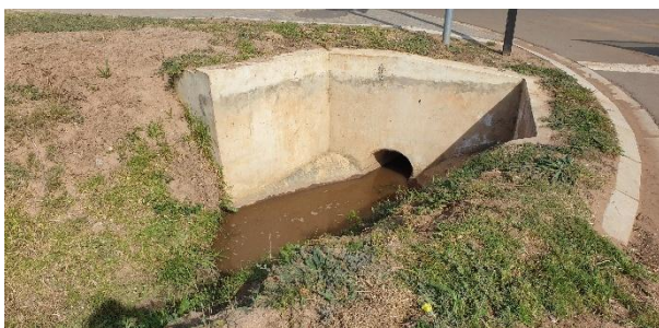
Stormwater inlet and outlet structure.
