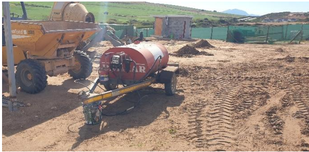
Fuel bowser available at the main site camp within Phase E adjacent to the N2.
