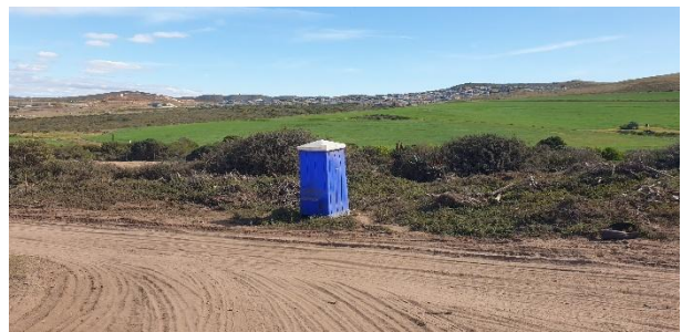
Chemical toilet in place where services area being installed in Phase D.
