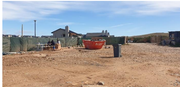
Condition of the construction camp adjacent to Erf 7380, skip is still available for waste management.
