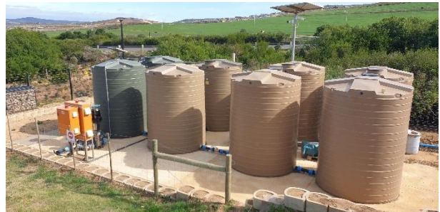
JoJo tanks installed on-site as backup storage for potential water shortages.
