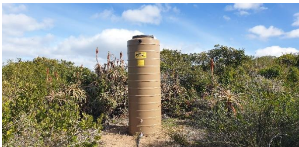
Jojo tank used for water storage for the bathroom at the guard building.
