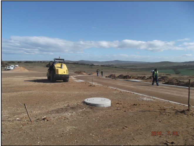
Image 5: Installed sewerage cesspit within the development site
