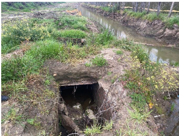
Collapsed culvert to be upgraded.
