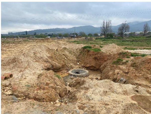
Civil service installations adjacent to the site camp.
