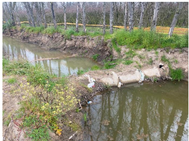
Recent rain filled the excavated stormwater channel; sandbags were placed to control flow.
