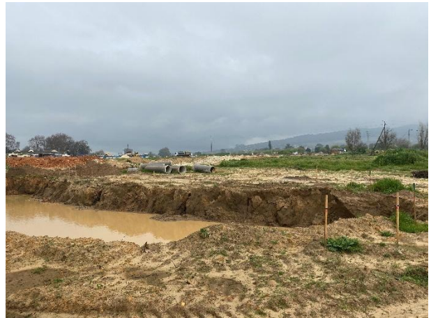
Smaller stormwater pond towards the north.
