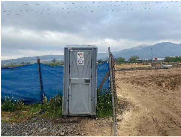
Chemical Toilet in place within the site camp.
