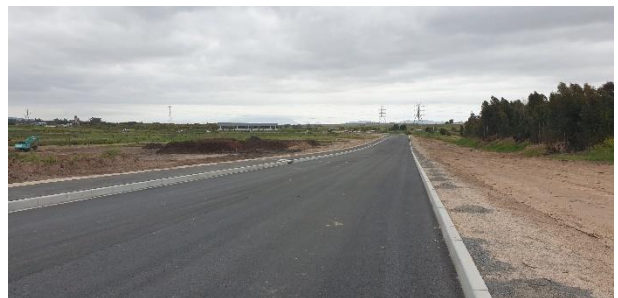
Condition of the main access road towards the west.
