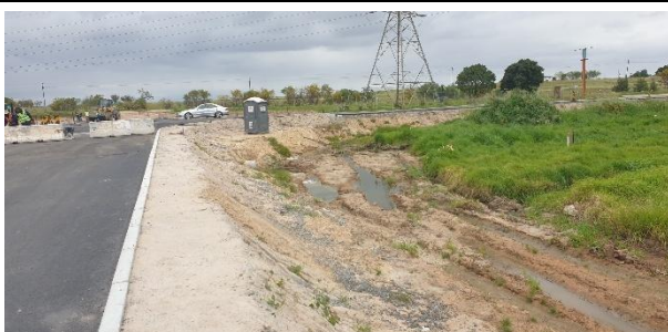
Condition of the drainage area adjacent to the main access road.
