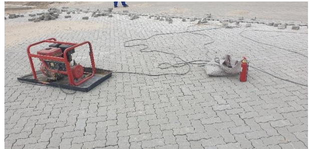
Generator placed within a drip tray, a fire extinguisher is present on-site.
