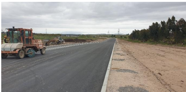
Condition of the main access road towards the west.
