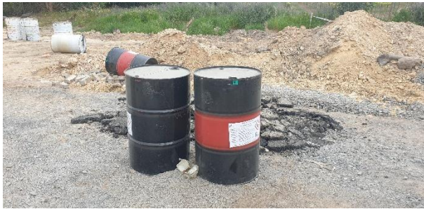
Empty bitumen emulsion cans located adjacent to the works area.
