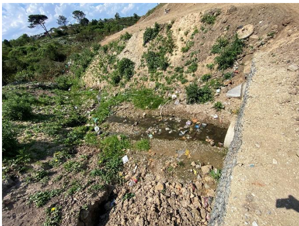
Upgraded stormwater outlet infrastructure. Erosion damage to be fixed and rehabilitated.
