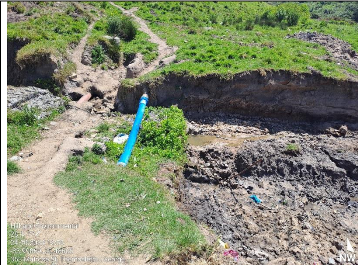
Existing services exposed and must be protected during construction phase.
