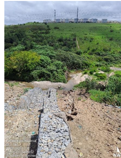
Erosion damage on the sides of the gabion structure will be backfilled and rehabilitated. Additional erosion protection to be installed (mulch sausages, sandbags etc). A gabion will be installed to prevent future erosion.
