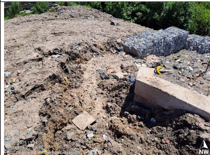
Construction progress (69a) – erosion damage to fixed and rehabilitated. Additional erosion protection (mulch bags or sandbags) to be used – where feasible.
