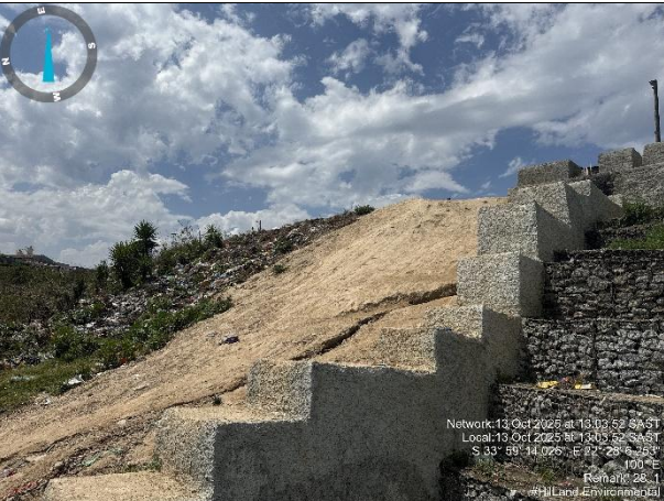
There are bare spots next to the gabion structure. Rehabilitation was damaged possibly due to high pedestrian traffic. The municipality can use excess topsoil from similar projects to replace on these bare spots.
