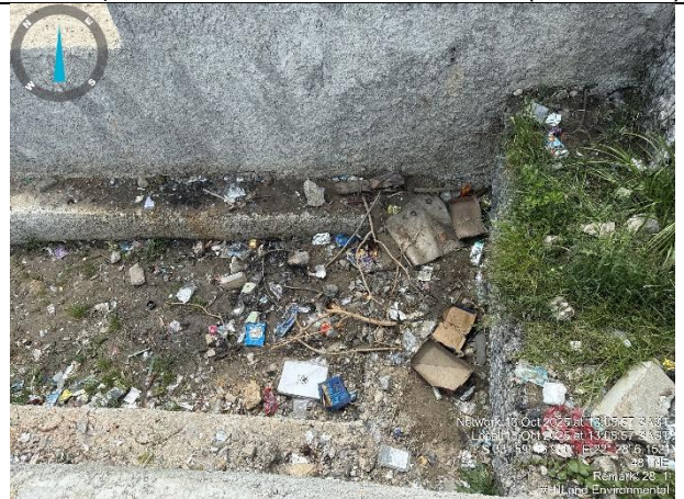
Litter in the stormwater network remains a problem
