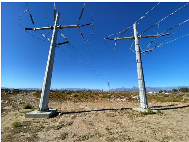
Completed Pylons 9 as seen towards the south. Significant dumping by the public occurs in this location.
