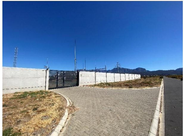
Entrance to the Transhex substation.
