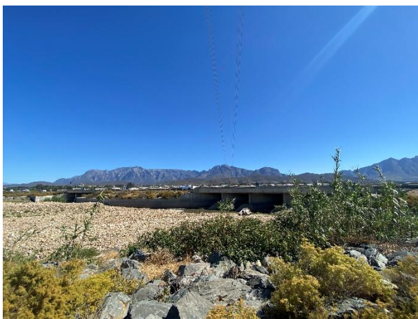
Condition of eastern bank of the Hex River at the R60 near Pylon 17 seen towards the northwest.
